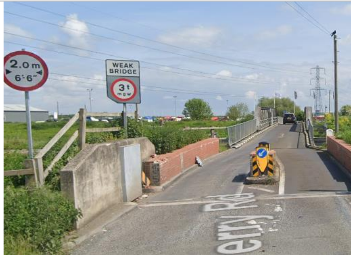
Plate 2-14: Weak Bridge on Ferry Road
