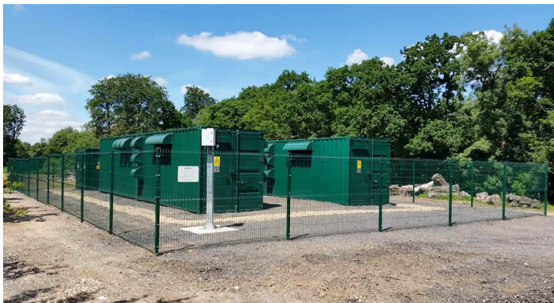
Plate 2-6: Typical Central Inverter and Combined Substation
