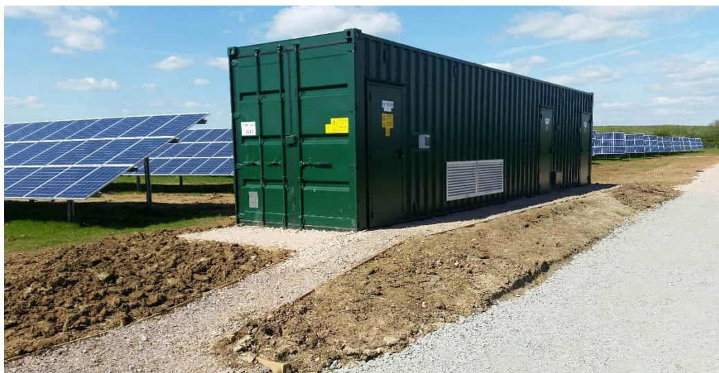
Plate 2-7: Example Field Substation
