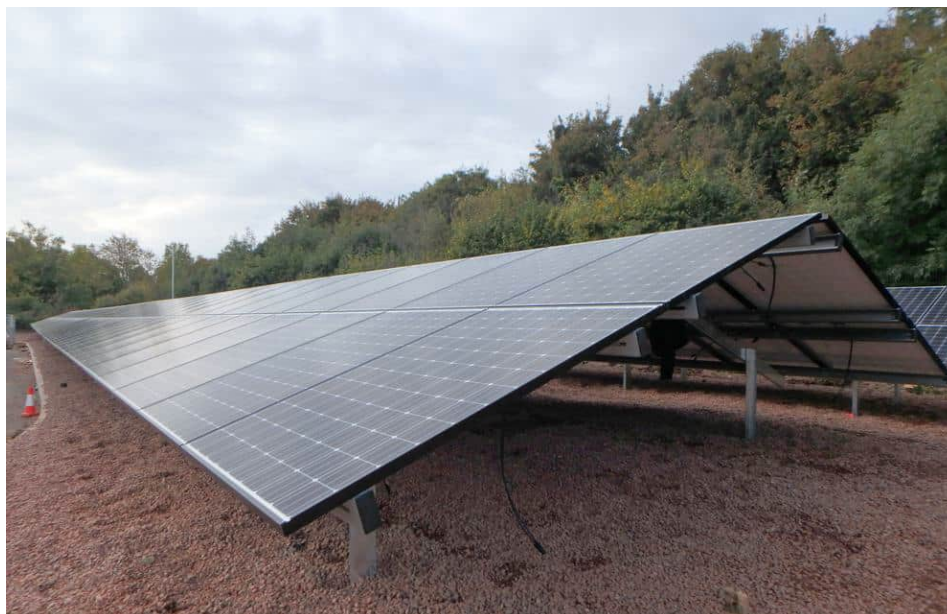
Plate 2-3: East-West Facing Fixed Tilt Modules, Finished Array
