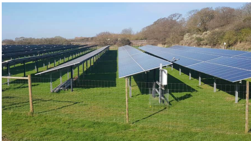
Plate 2-2: South-facing Fixed Tilt Modules, Finished Array
