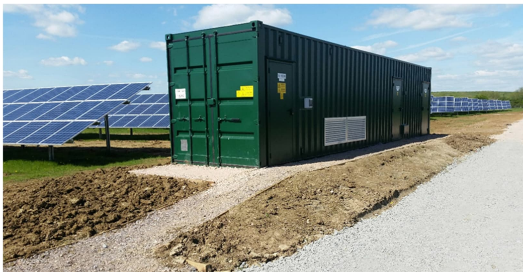
Plate 4: Typical Unit Housing the Transformers and Switchgear
