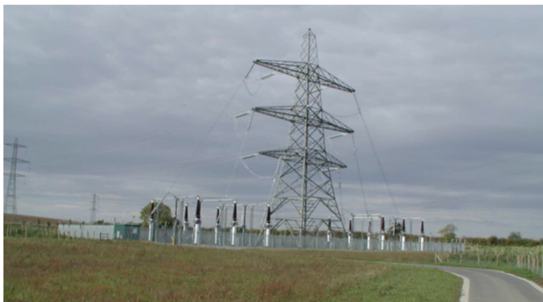
Plate 2-6: Example Line Drop On-Site Substation
