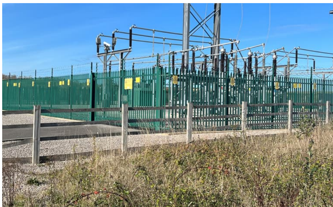
Plate 2-5: Example On-Site Substation showing Infrastructure and Fencing
