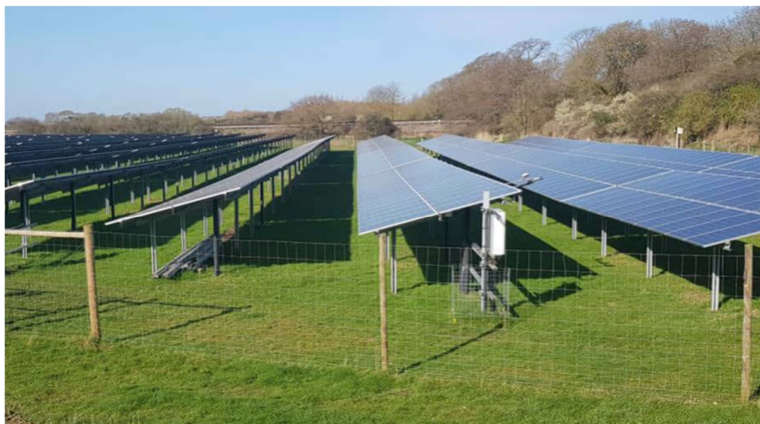
Plate 2-2: Example South Facing Solar PV Panels
