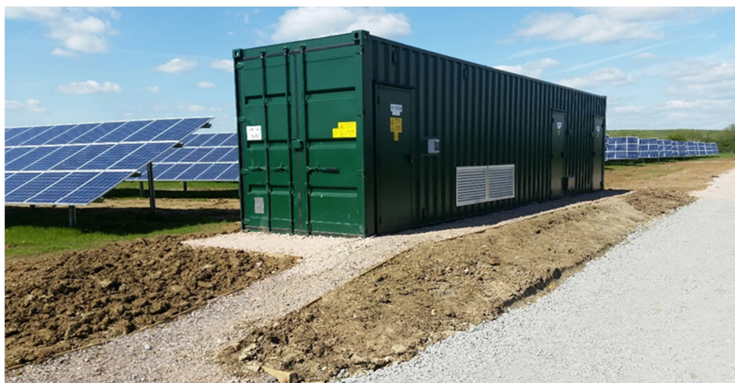
Plate 2-4: Example of a Field Station Unit
