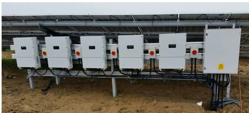
Plate 2-3: Typical String Inverter Installed Next to Solar PV Panels
