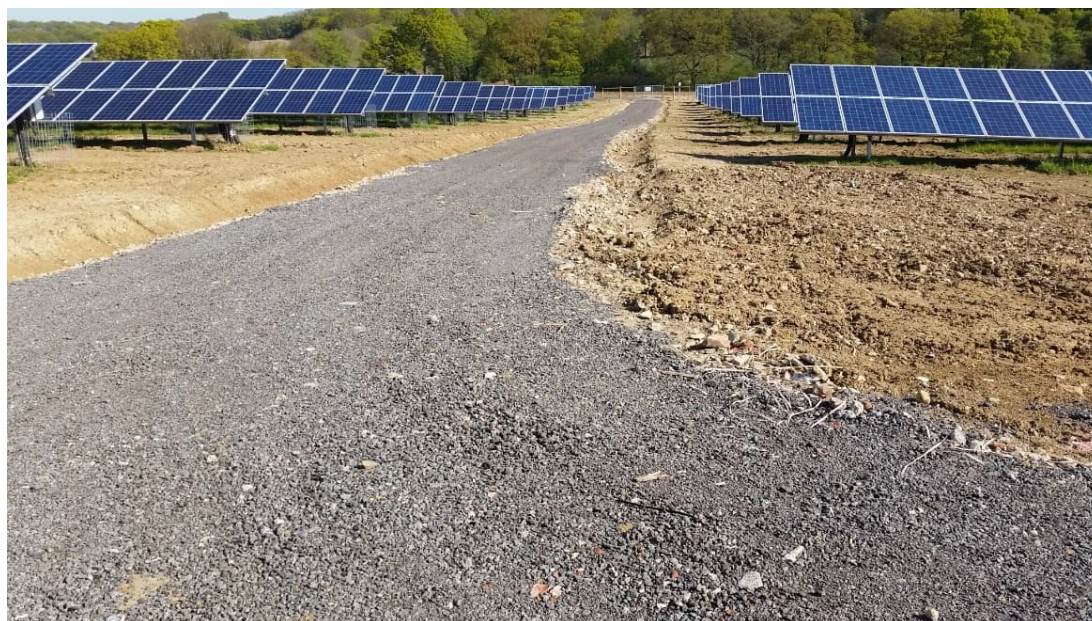
Plate 2-10: Typical crushed stone access track laid on hardcore and geotextile (photo during construction phase and prior to landscaping)
