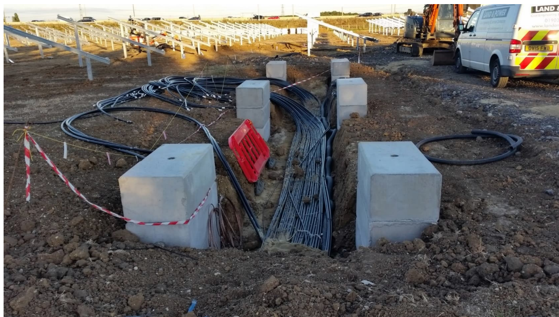
Plate 2-13: Example Underground Cable Installation Beneath a 33 kV Field Station Unit Awaiting Delivery
