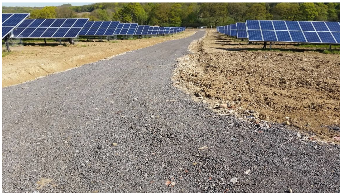
Plate 2-14: Typical Crushed Stone Access Track Laid on Hardcore and Geotextile (Photo during Construction Phase and Prior To Landscaping)
